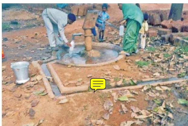
Water and garbage spreading and cracked drainage of the source (Handpump near Mahila Samiti, slum Vijonagar Joaklandi)
