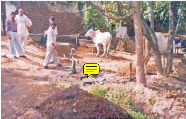
Handpump with no apron, presence of animal waste around the source
