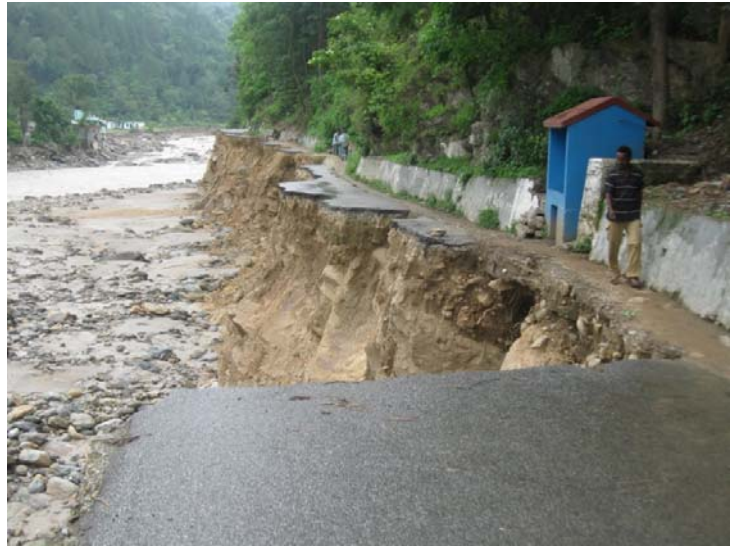
Destruction of National Highway to Kedarnath (2)
